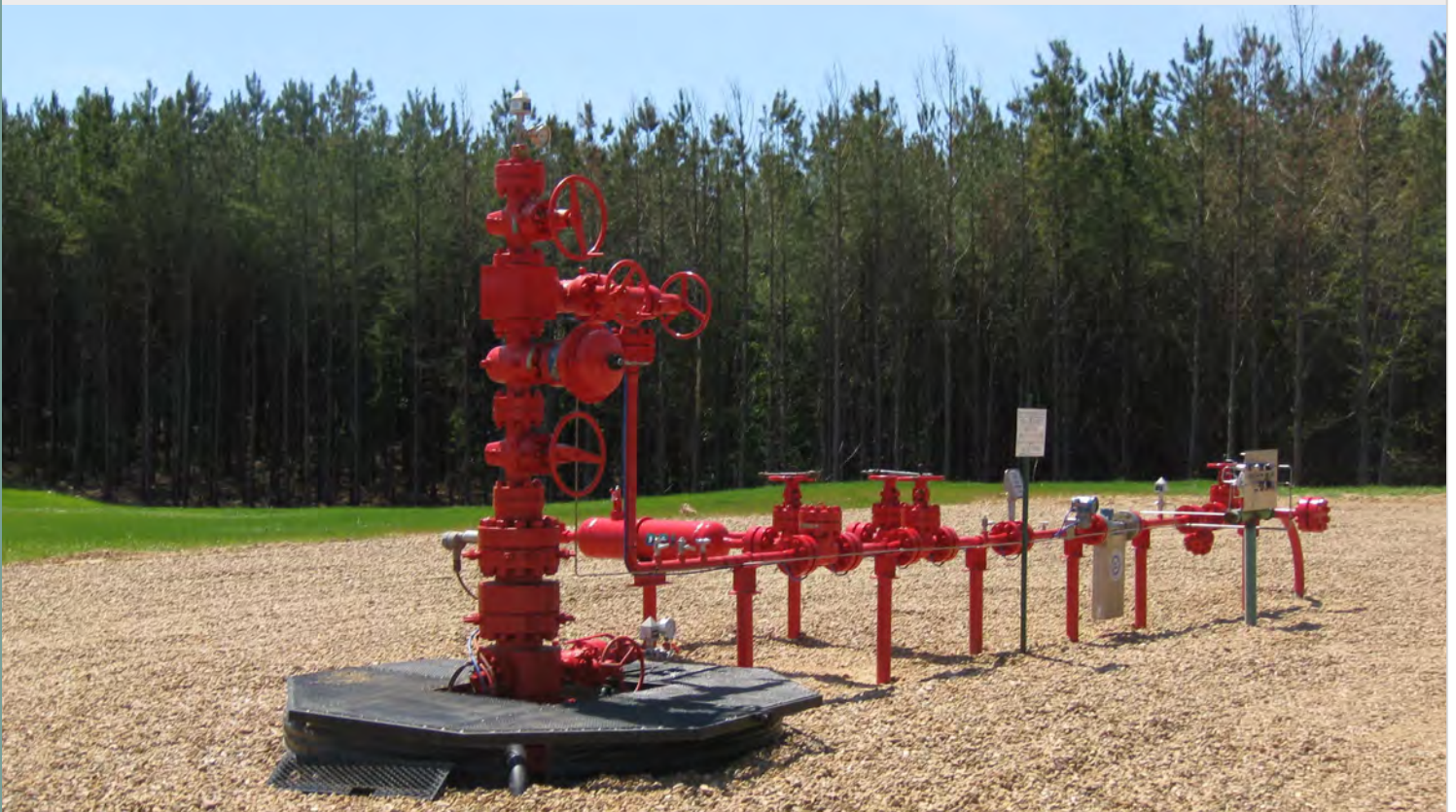
A carbon dioxide (CO 2 ) injection well drilled by the Southeast Regional Carbon Sequestration Partnership (sponsored by the U.S. Department of Energy) at the Cranfield CO 2 test site in Mississippi. Source: Geology, Energy & Minerals Science Center, United States Geological Survey. https://www.usgs.gov/media/images/co2-injection-well-mississippi . 2010.
